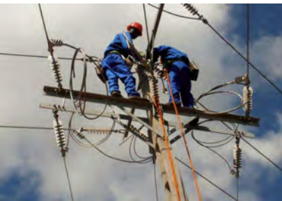
Electricity III, Inhambane Mozambique
