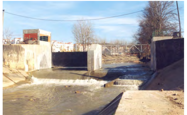
Inflatable at Arrabalde: view downstream of the two spans, cofferdam and house to electrical controls
