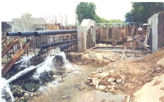
Inflatable weir at Arrabalde: river to flow only in the lower tubes, during the execution of work
