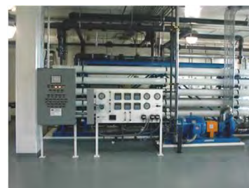
Diversas vistas do equipamento instalado na central. Several views of the equipment installed in the facility.
