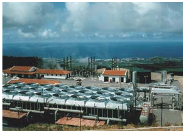
EDA - Geothermal Plant at Ribeira Grande S. Miguel - Azores
